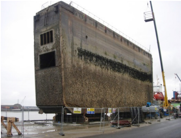
One of four 800-ton lock gates used to maintain water level on the tidal river at the Chatham Dockyard, in the UK.
